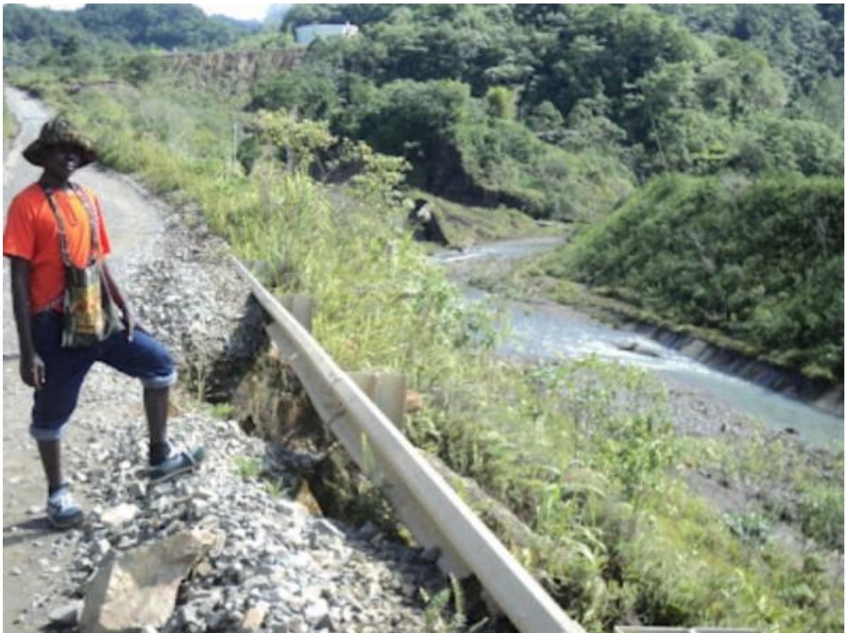
Landslide affected zone of the Kavarong waterway near the BCL concentrator
