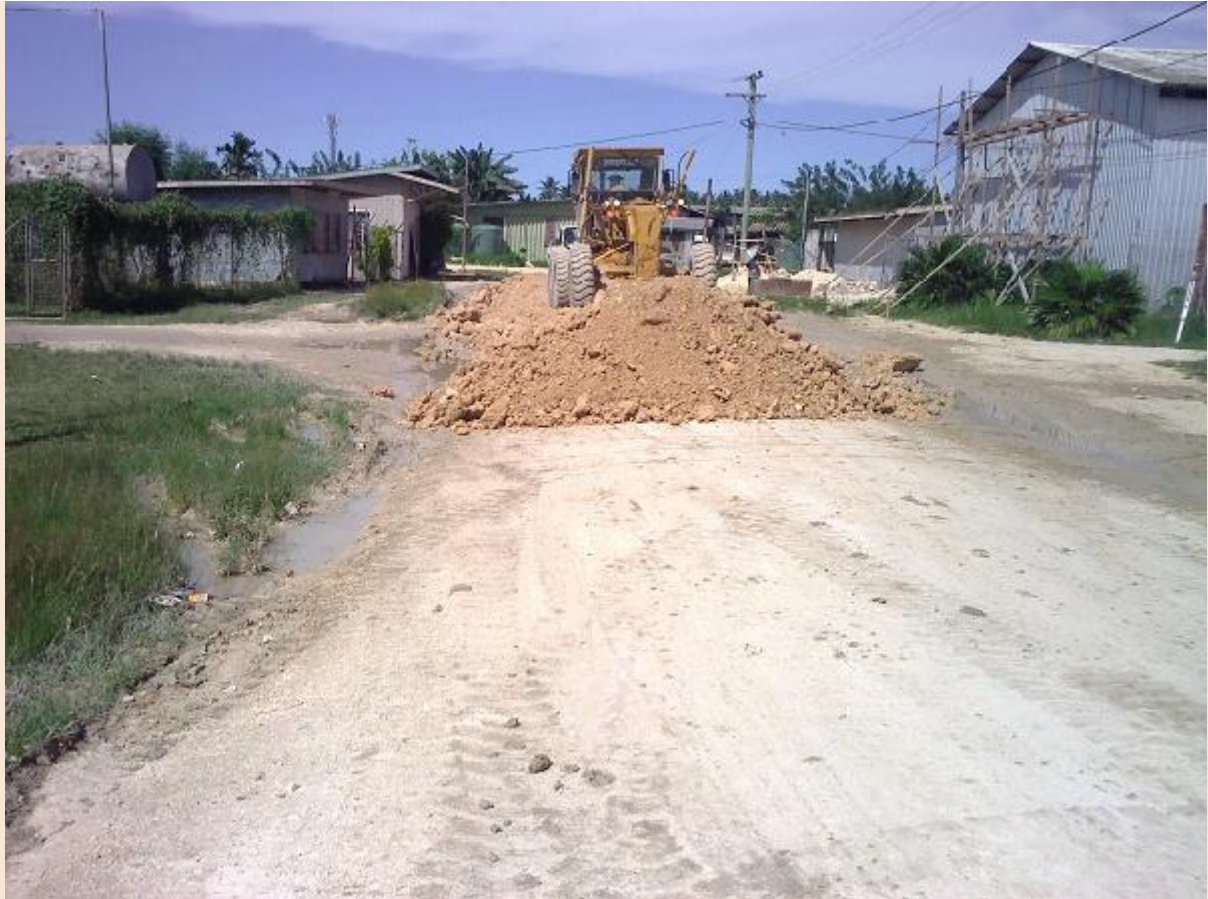
Pictured are workmen upgrading the stretch of road between BMF and Mark Murava building on the back street.
